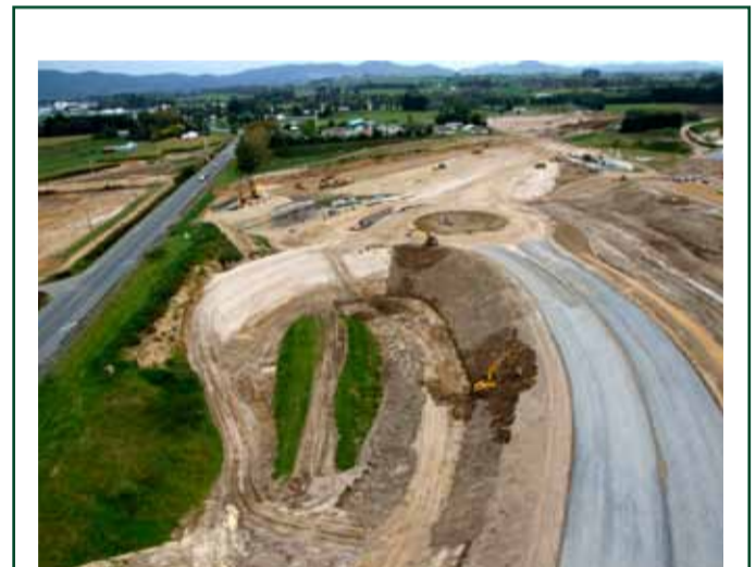
Roundabout adjacent to SH1 showing Stevenson aggregate laid on the new road (on right)
