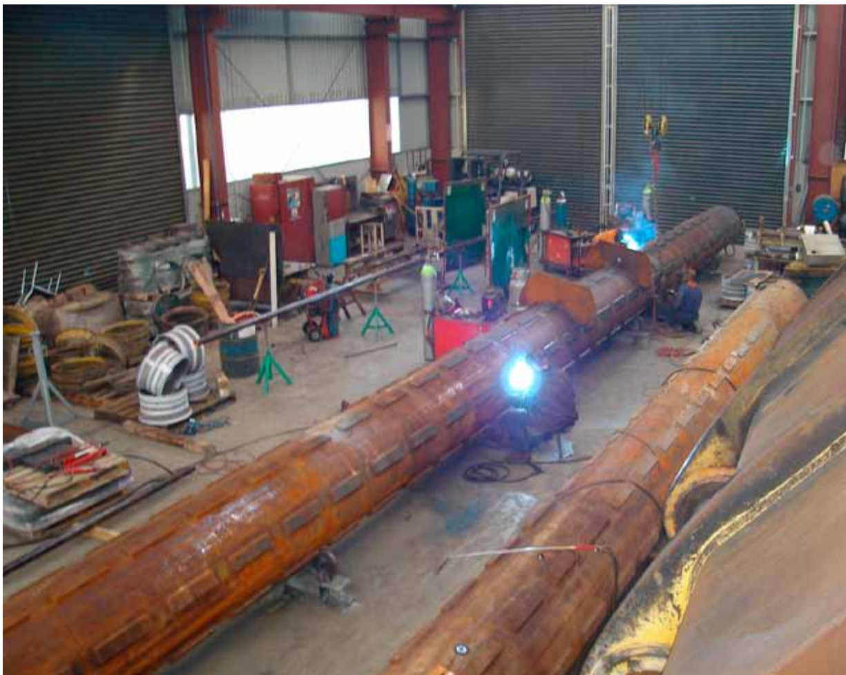
Spud legs in Stevenson Engineering's weld shop in the process of being repaired and extended.
