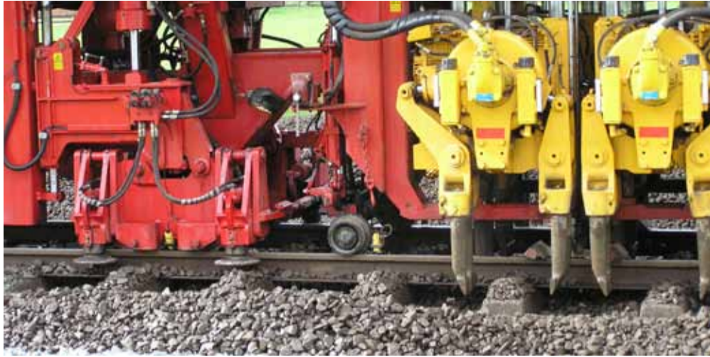
KiwiRail ballast train in action. Left - the rail track is lifted to the correct level as on the right, tines prepare to vibrate and tamp down the ballast rock into position.
