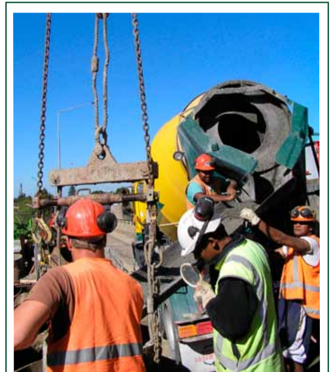
GHP Piling and Stevenson filling piles on the Market Road to Greenlane lane extension project
