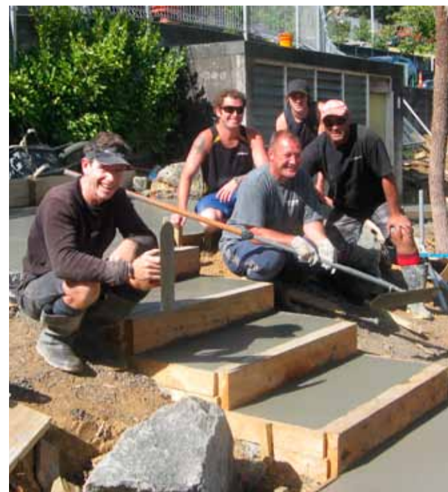
The volunteer team rests after placing Stevenson Concrete's 16mm Hawkes bay pebble with steel trowels. L-R front: Dean Lawson, Custom Concrete, Brent Atkinson, Stevenson Concrete, Phil Opetaita, AAA Pumps. L-R back: Dan McKay and Luke Jelly, Palmers, Remuera.
